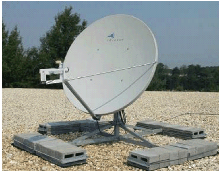
Figure 7 Typical Antenna with BUC and LNB
