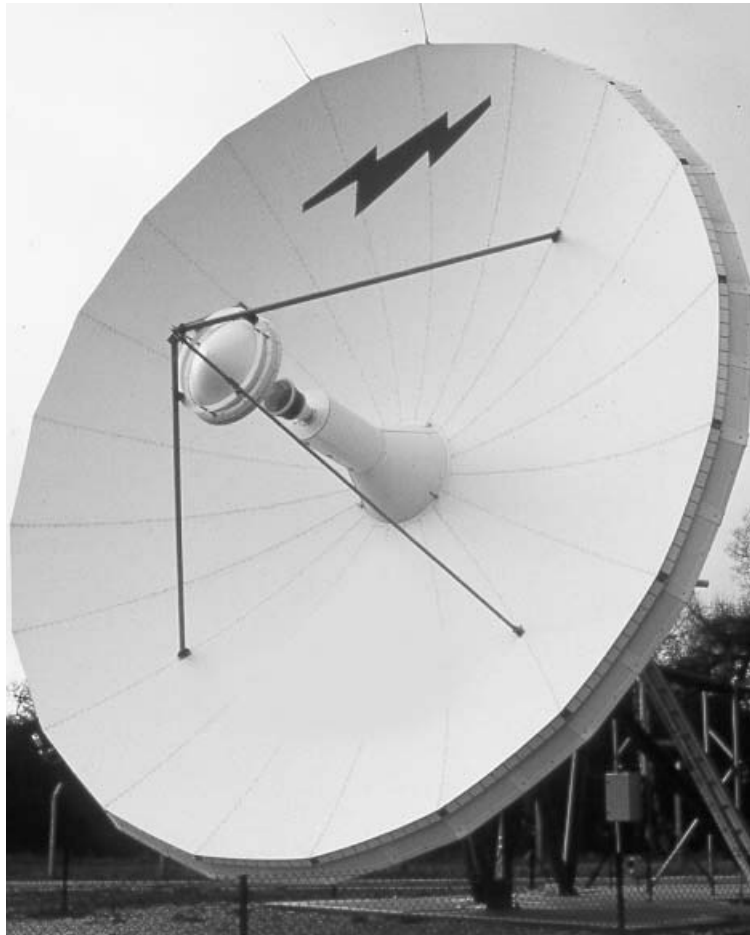
9.3-Meter Earth Station Antenna
